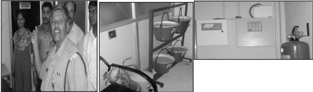
FIRE & BURGLAR ALARM SYSTEM, AUTO-DIALLER SMOKE DETECTOR, MOTION SENSOR MANUAL CALL POINT, ALARM HOOTERS
