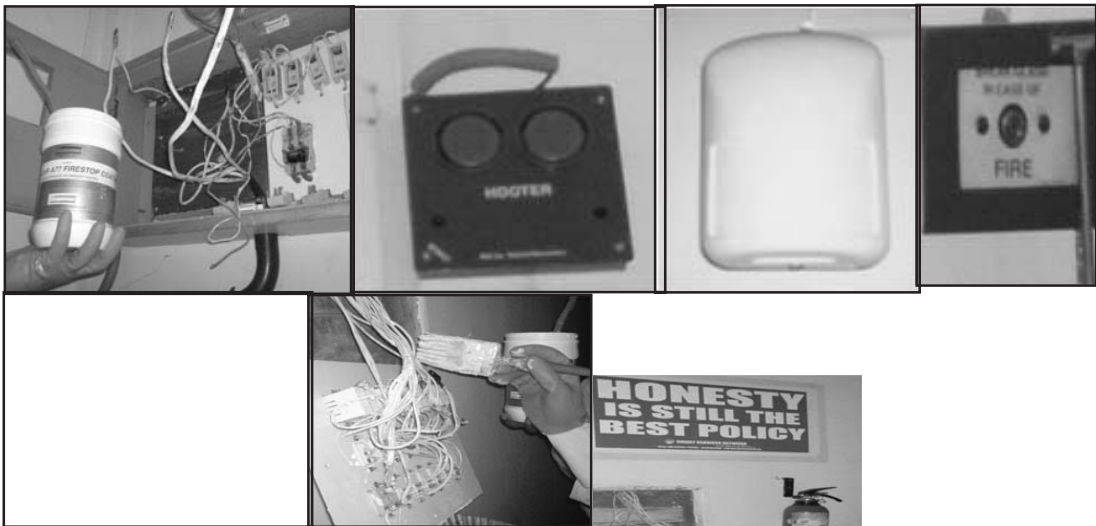
FIRE SUPPRESSORS - IMPORTED CHEMICAL FROM GERMANY - APPLICATION AT ALL TERMINATIONS TO AVOID ELECTRICAL SHORT-CIRCUITS (PREVENTIVE MEASURES).
