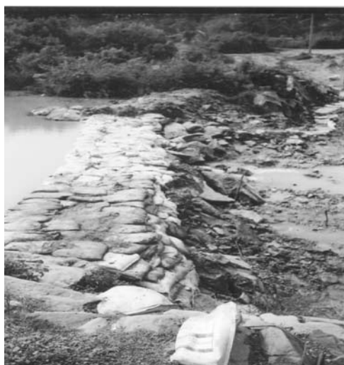
Breaching of embankment due to flood
